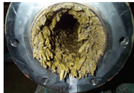
Fig.8: Gravity Concentrated Sludge Pipe Wall
