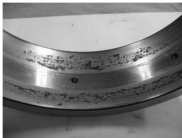
Fig. 7 Example 1 (33rpm/E_area=3,584) : (upper) measured AE waveform and periodicity spectrum, which reveals outer-race damages, (lower) photo of the removed bearing; terrible flaking on the outer race as well as damages on the inner race and rolling elements were observed.
